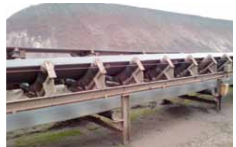
This roller bearing is overheated and should be replaced.
